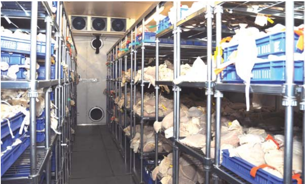
Figure 4C.1.2. Walk-in seed drying room at ICRISAT genebank.
